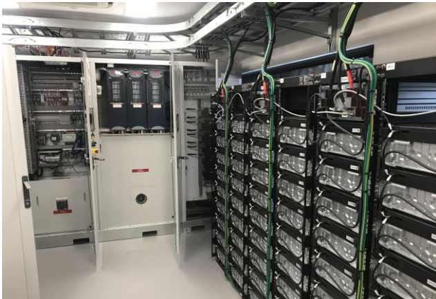
Fig. 1. Indoor energy storage system, electrical and control cabinets hosting 300 kVA grid-forming converters and 500 kWh li-ion battery racks (right).
