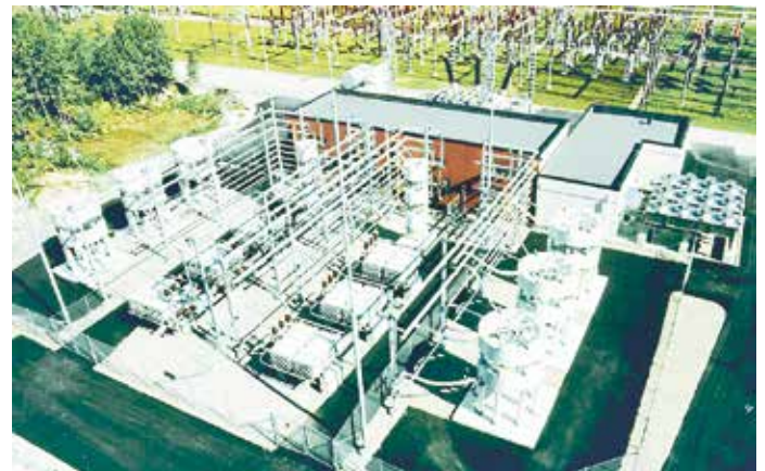
The SVC is an excellent tool for achieving dynamic voltage control of power systems.
