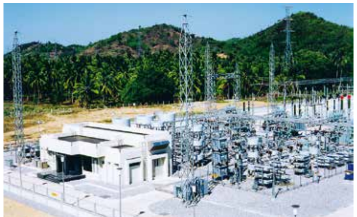
This SVC has boosted power transmission capacity by over 50 percent in a 230 kV system.
